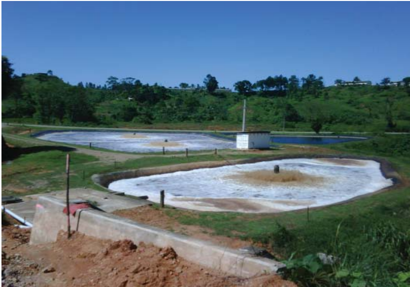
Figure 5: Naboro Landfill leachate treatment system after aerators installation.
