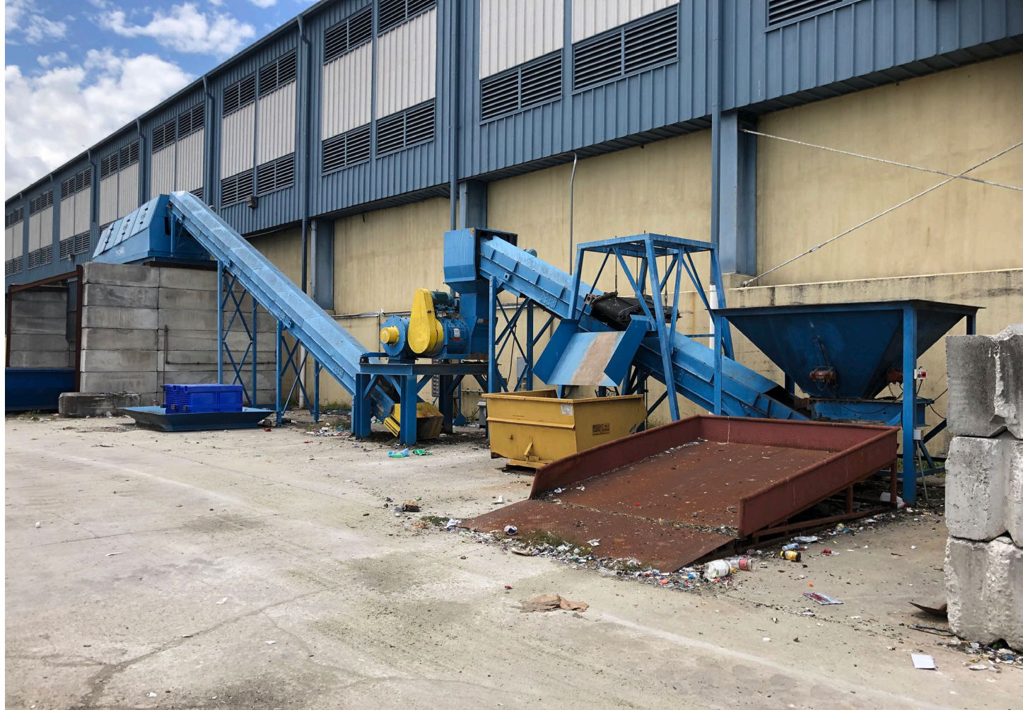
Primary Glass Crusher System
