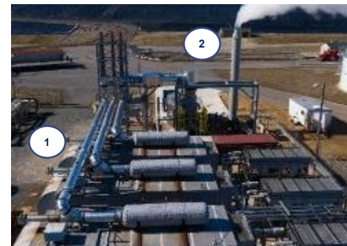
(1) Exhaust gas is ducted together to provide thermal energy for evaporation (2)
