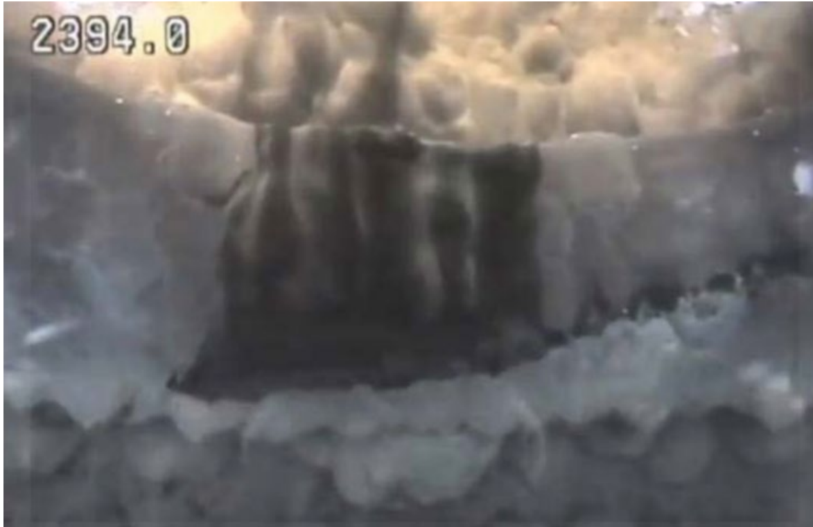
Bottom of the 6.21-inch FRP
