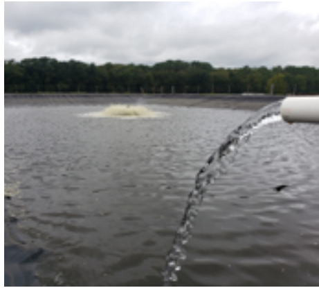
Treated Leachate Discharge and Storage.
