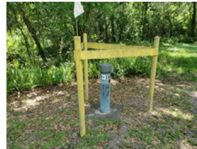
Typical groundwater monitoring well at a Florida landfill.
