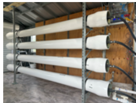
Reverse Osmosis Membrane Vessels.
