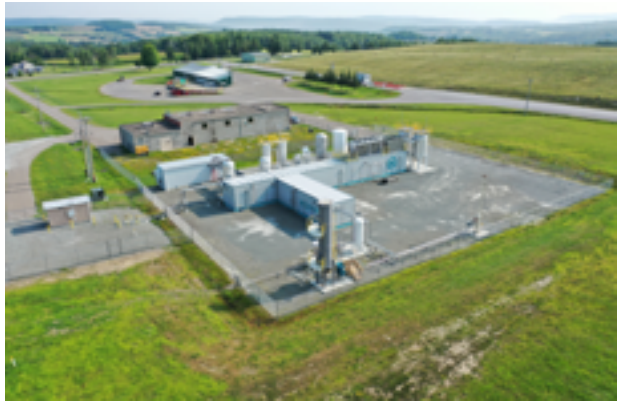
The WAGABOX® Facility in Steuben County, NY.
