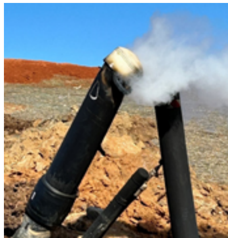
Figure 2 - Subsurface fire due to compromised infrastructure.
