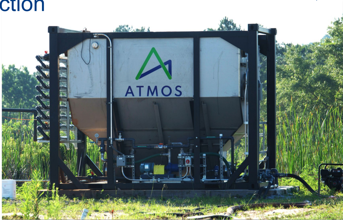
Gravity Clarifier TSS reduction
