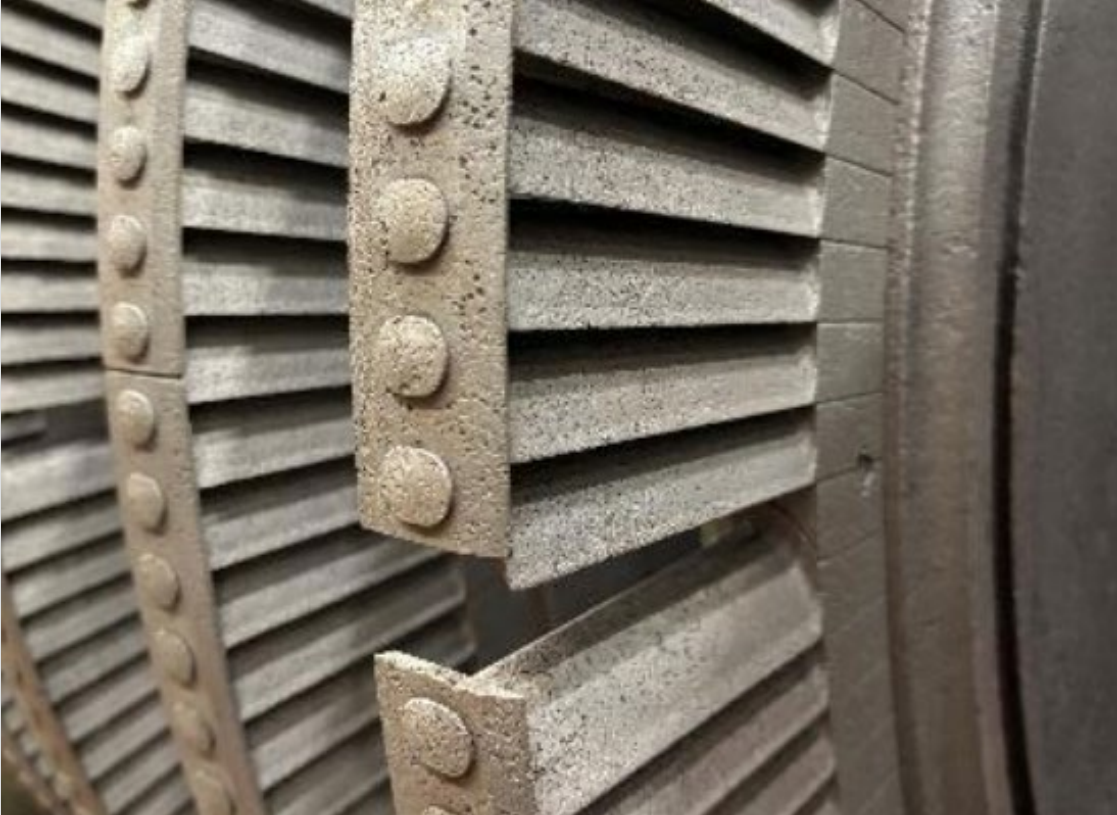
Stage 8 Buckets/Tenons – Heavy Pitting/Erosion
