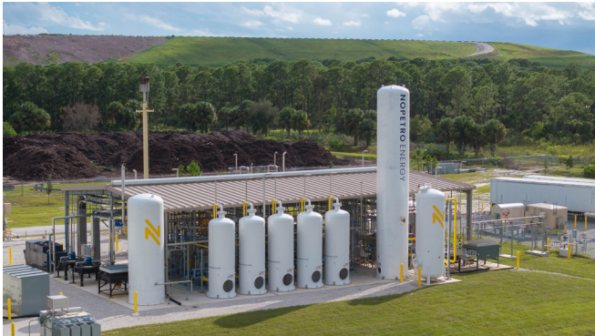
Nopetro Energy’s Vero Beach Facility removes CO2 to produce methane of over 95% purity, exceeding fueling standards. Courtesy of Nopetro.
